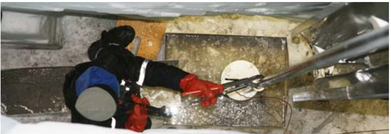
The rock drill extension is now so long that the last rod has to be mounted with the drill in vertical position. An unusual operation that needs to be carried out at the bottom of the inclined drill trench. There is a high risk of drill liquid showers.
