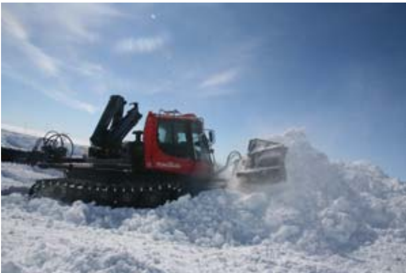
PistenBully in action moving snow from south side of the drill trench
