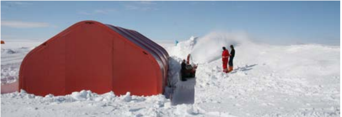
Garage: Substantial excavation is needed to free the garage from the grip of snow. This garage was built on a 1.5 m hill in 2008.
