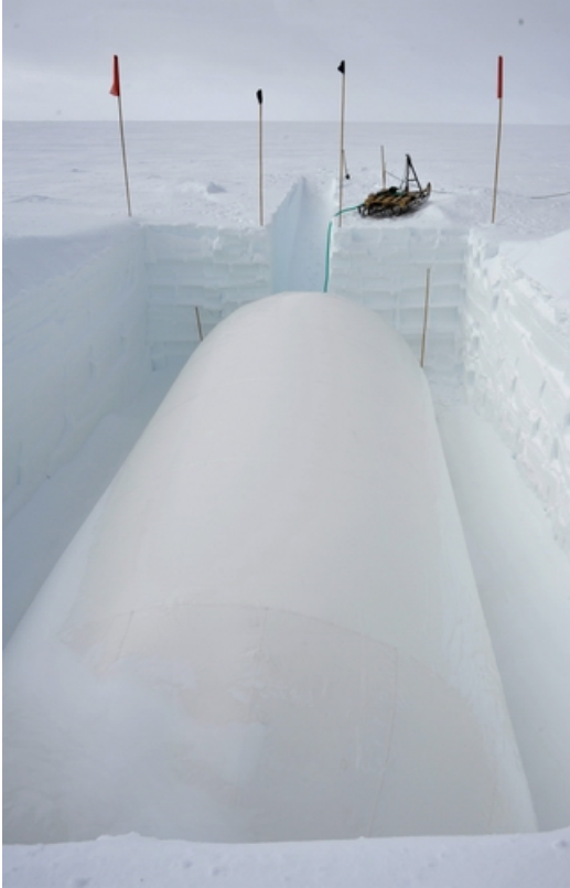
Balloon: A view of the 15 m long and 4.85 m wide gas tank in the trench before we began to bury it.
